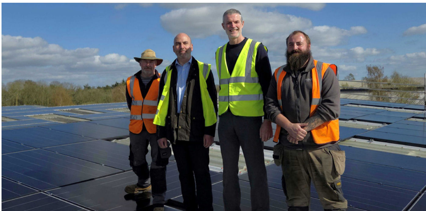
Solar installation at Wrightfield
