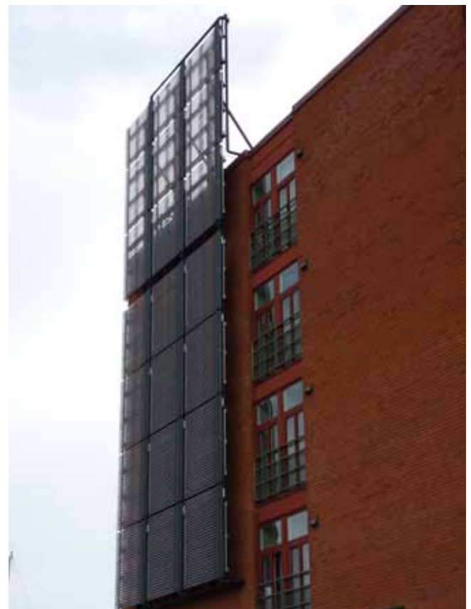
IMAGE OF A SOLAR THERMAL ARRAY CONNECTED TO A DISTRICT HEATING NETWORK IN MALMÖ, LDA DESIGN, 2011
