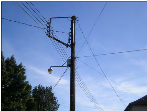
(Fig 57) Unsightly wirescape in The Street
