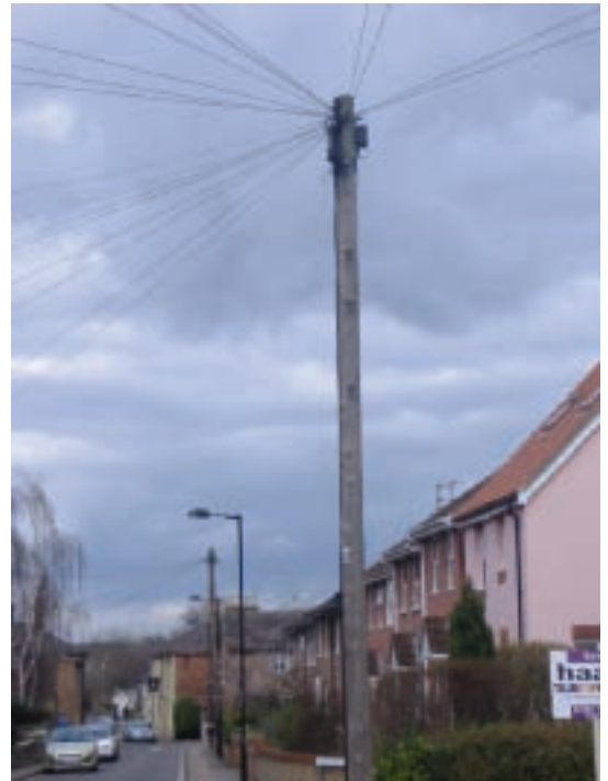
Photo 65: example of overhead wires in the conservation area
