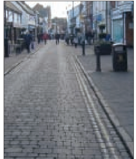
Photo 38: Tumbled blocks to carriageways
