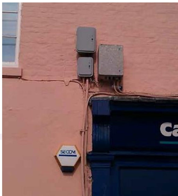
Alarm boxes can be conspicuous and should be positioned as discreetly as possible
