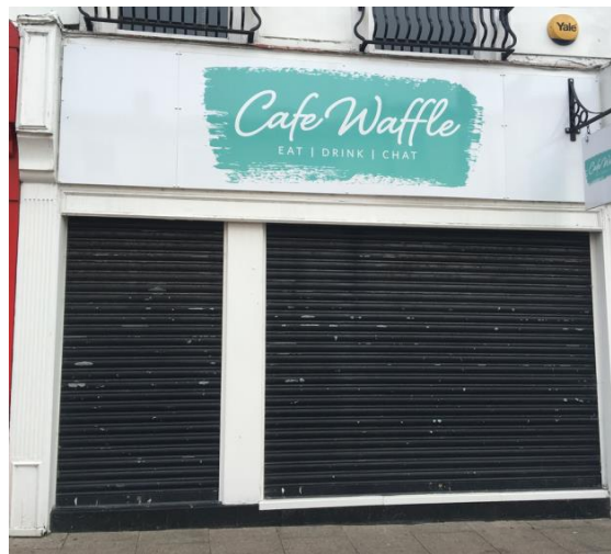
Visually harsh and unsympathetic external roller security shutters
