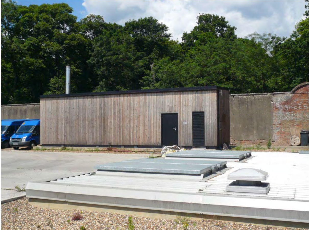
5: New wood chip biomass boiler adjacent to the Sports Centre, opened in 2012. This is a key part of the School's commitment to sustainable management practice. See paragraph R4.2.9.
