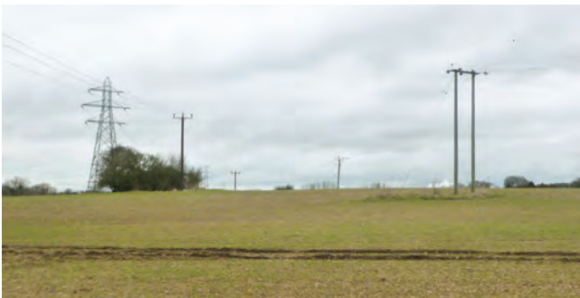
132kV, 33kV and 11kV overhead lines
