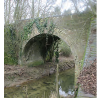
Bridge over the River Lark remaining from the dismantled Bury St Edmunds to Long Melford railway line
