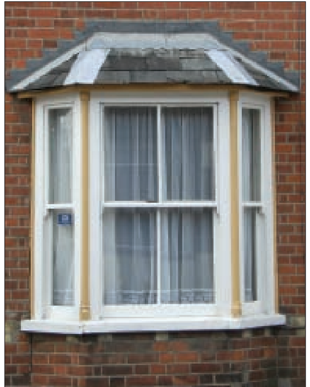
Photo 14: Original bay windows provide additional space and are an important characteristic to the terraces of Mount Road
